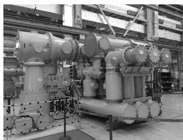
图13 整间隔局放试验 Fig. 13 Partial discharge test of integral interval
